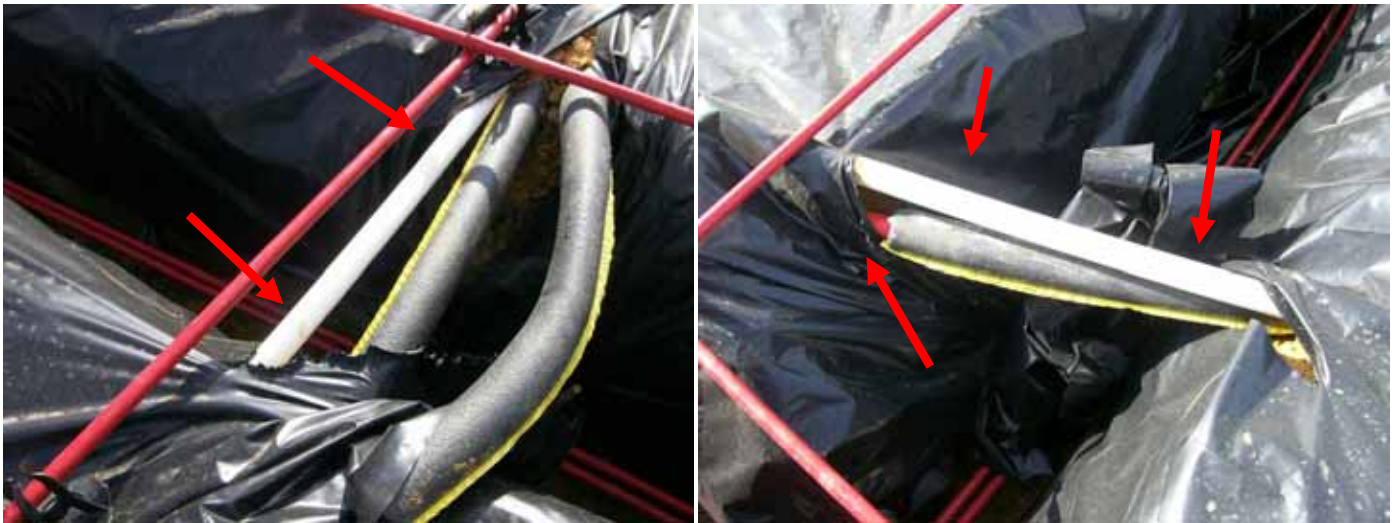
The plumbing needs to be covered with insulation.
