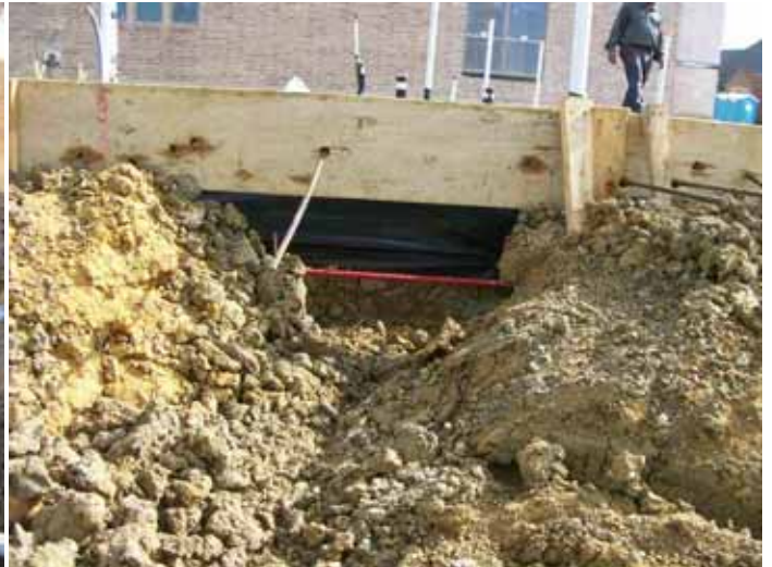
Fill needed against the former boards.
