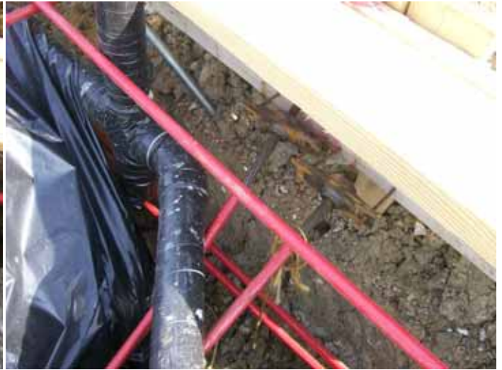
Cable ends need to be wrapped. Plumbing lines need to be insulated.
