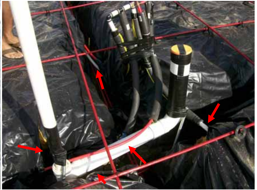
The plumbing needs to be covered with insulation.
