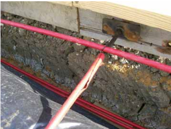
Cable ends need to be wrapped.
