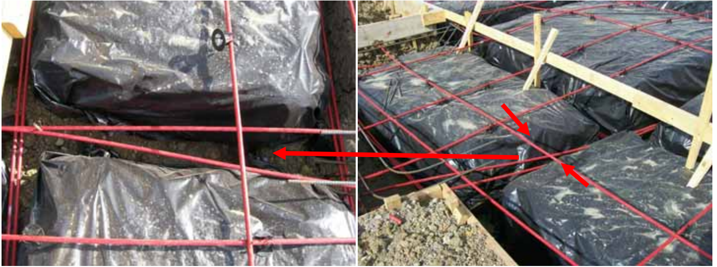
The beam needs to be widened in the front porch area.
