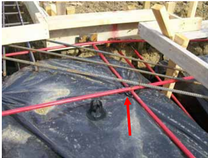
Chairs are needed under the cables and steel near the back porch area.
