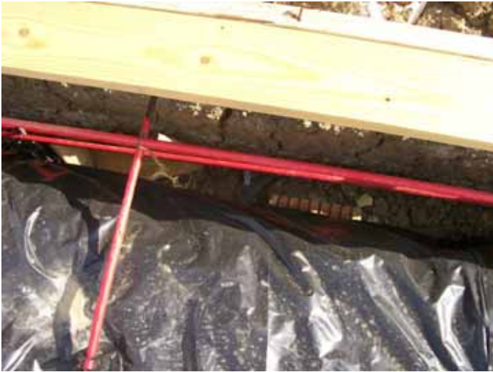
Debris needs to be removed from the crawl space.
