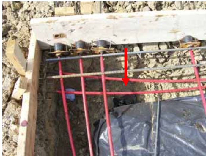
It is recommended to have two additional steel rebar strands in the beam footer at the front porch.
